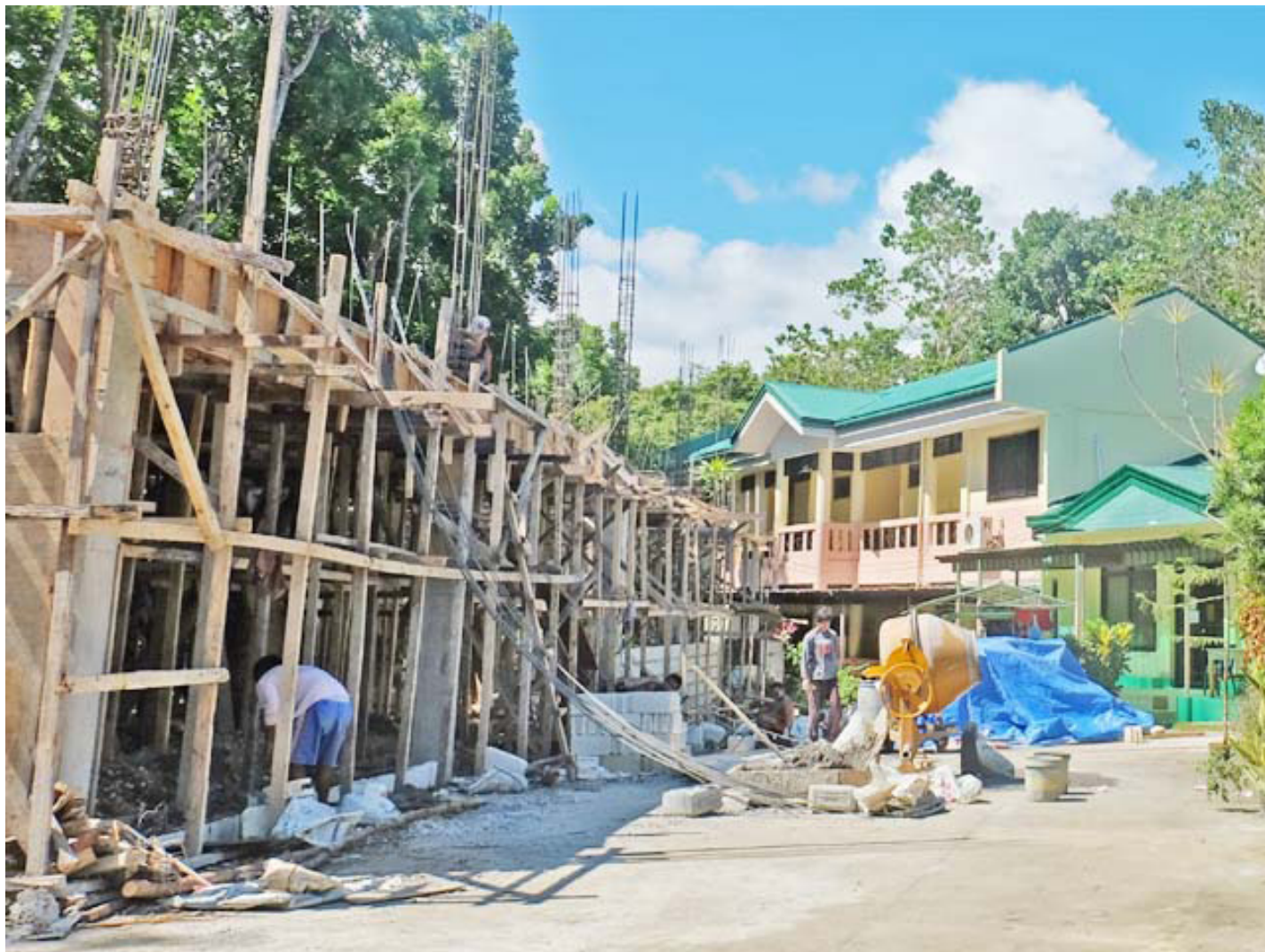
The on-going construction of the 4.6M budget two-story building of ATI-RTC 7 by Cempron Construction
